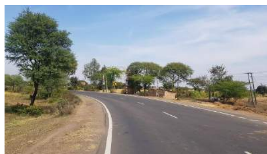
Km. 4+00 Chevron signs on the curve section
